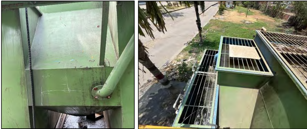
TUBE SETTLER: BEFORE MODIFICATION
