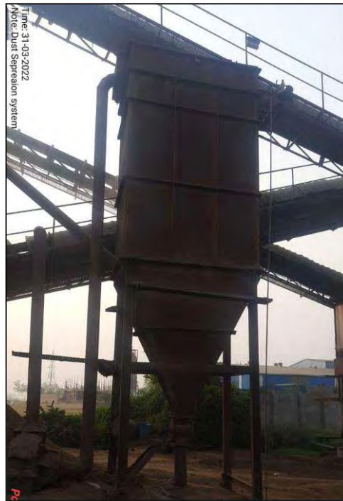
Dust Suppression System
