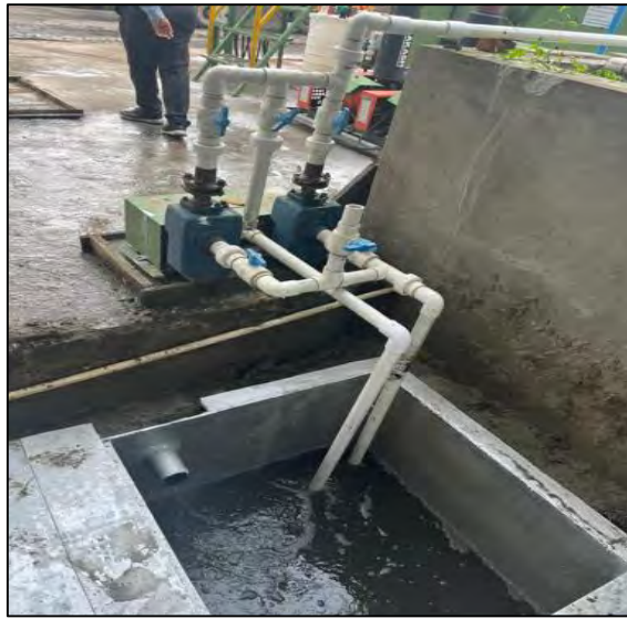
FLOW METER AT INLET TO MAINTAIN THE FLOW OF SEWAGE
